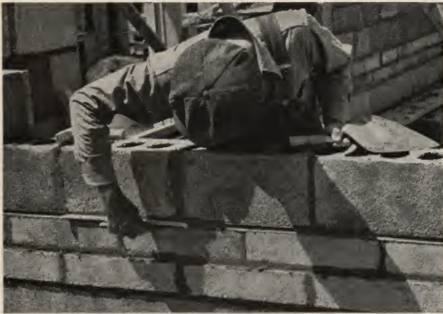
2—Mason grooves the mortar with a round tool to emphasize the horizontal joint.
